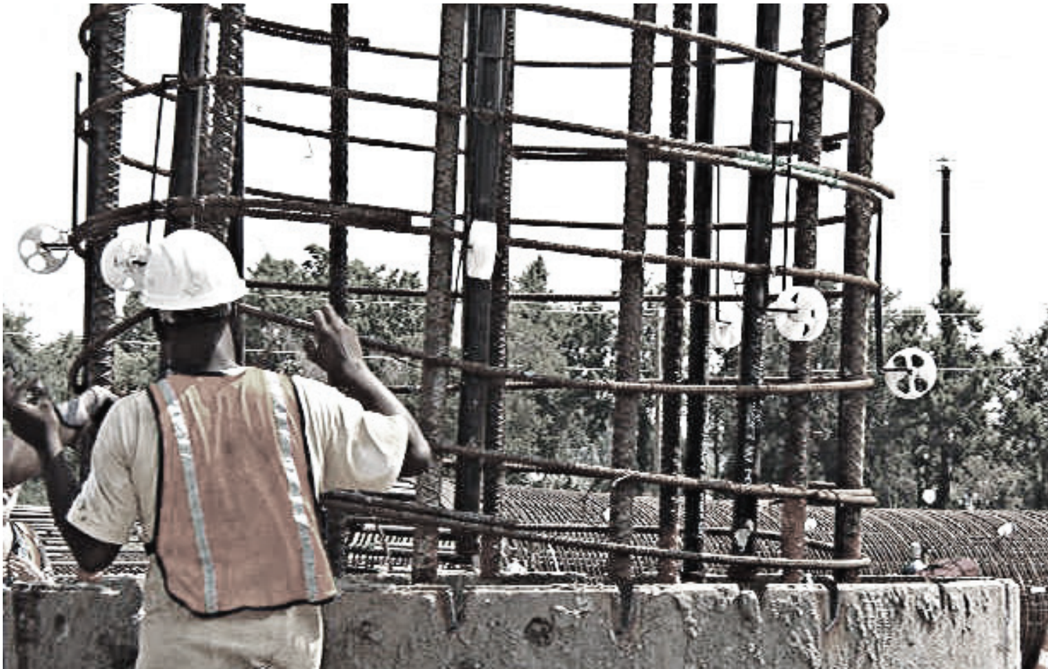
Guiding rebar cage into drilled shaft with Hairpin and ShaftSpacer system attached
