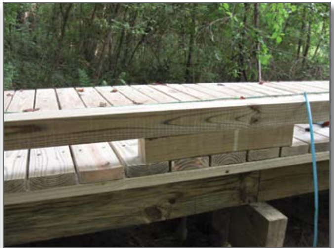
Step 9—Curbing (6 inch by 6 inch or 4 inch by 4 inch, depending on the width of maintenance equipment using the boardwalk) on top of scupper blocks is specified in lieu of railings for this OHV trail.
