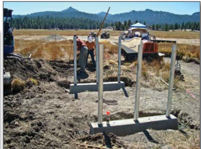
Step 4—The substructure is placed on top of the wrapped geocell filled with gravel so it is flush with the final ground elevation. Two Manta Ray earth anchors are installed for each precast concrete foundation to restrict uplift and lateral movement.
