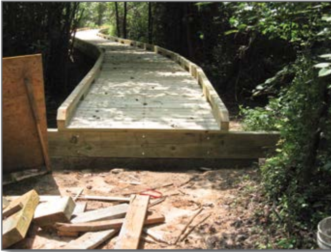
Step 10—Backwall planks installed at the end of the boardwalk keep dirt from sloughing between the beams and prevent moisture from wicking into the ends of the beams.
