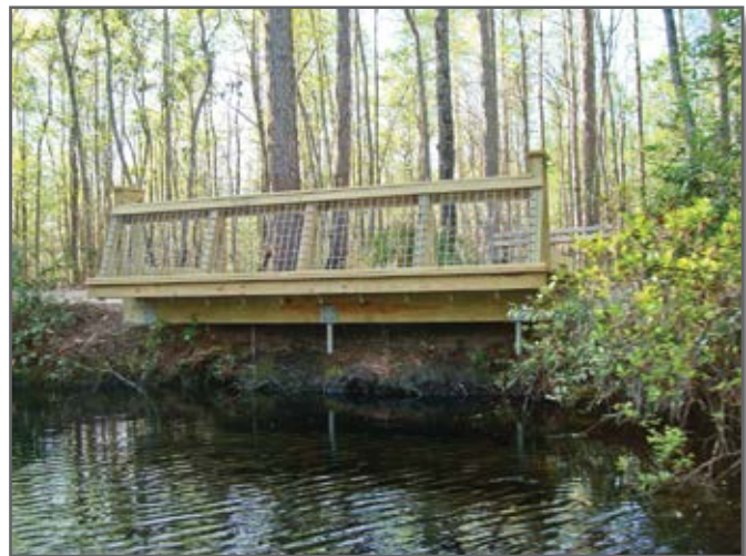
Figure 1—Helical piles support this viewing/fishing platform at the Okefenokee National Wildlife Refuge in Georgia.
