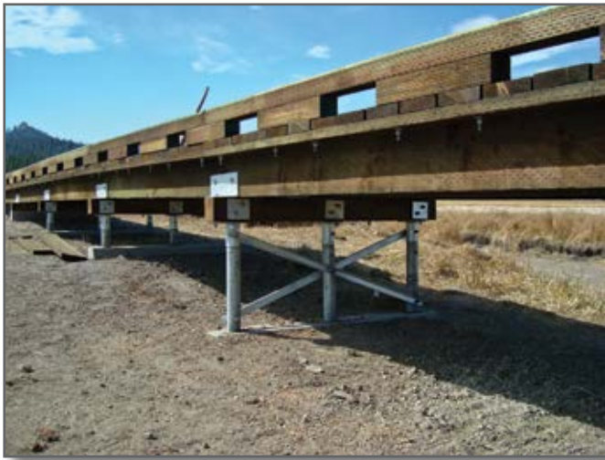
Step 11—The finished structure features curbs with scupper blocks for this all-terrain vehicle/motorcycle trail.
