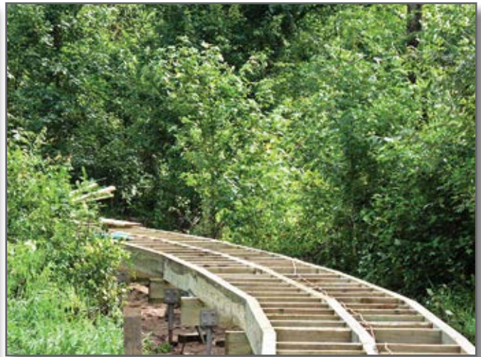
Step 8—Bracing is added between the stringers to prevent the stringers from rotating.
