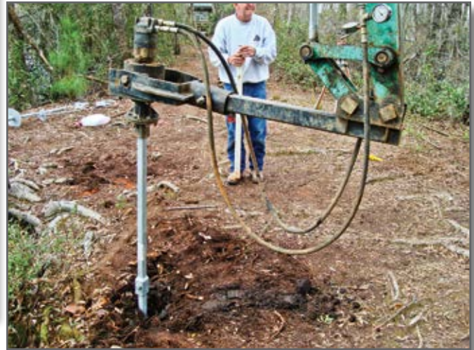
Figure 4—Specialized equipment is needed to install helical piles. For this installation, Trails Unlimited installed 12 helical piles for 4 viewing platforms in 4 hours.
