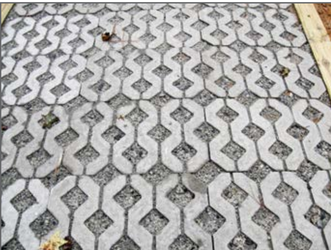
Step 12—A closer view of the Perstone pavers used in the installation.
