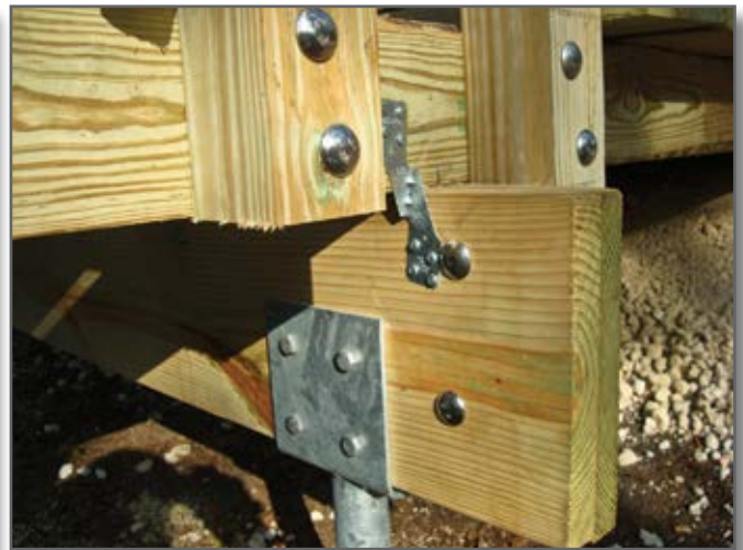
Step 6—Simpson Strong-Tie metal components are used to tie down the joists to the header beam.
