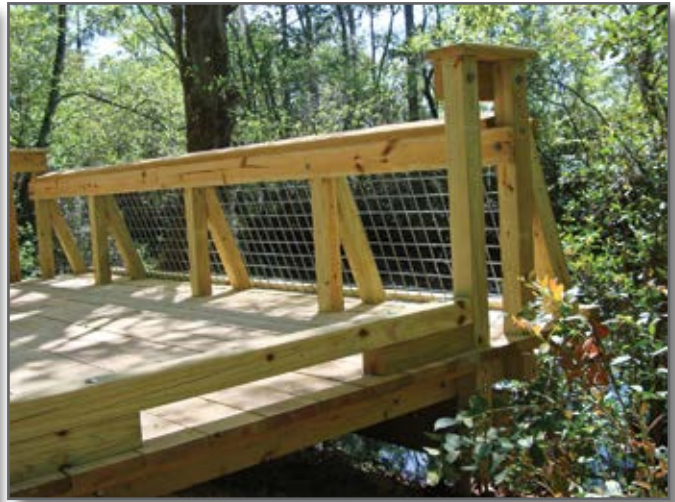
Step 9—The front handrail is sloped to allow the legs and front wheels of a wheelchair to be positioned slightly underneath the top rail. The handrail height is 34 inches. Welded wire mesh is installed to discourage alligators from using the platform, to provide better views of the canal channel scenery, and to prevent small children from falling in the water.
