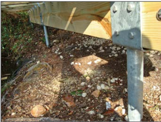
Step 4—Saddle brackets are bolted to helical piles to support the header beam, forming a bent. In this case, the timbers are alkaline copper quaternary (ACQ)-treated southern yellow pine.
