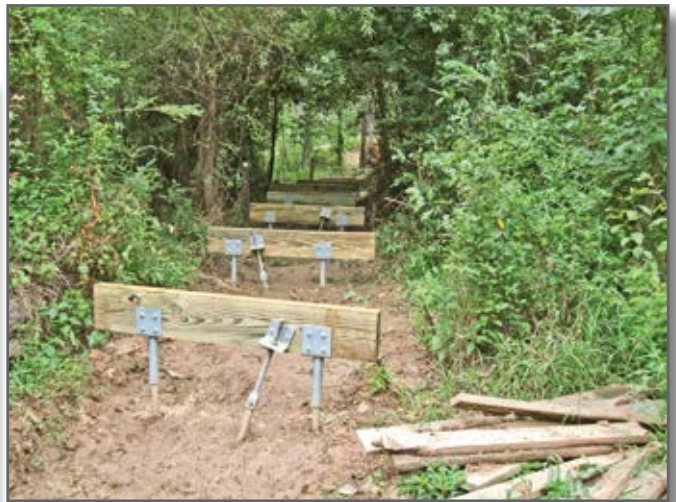
Step 5—Header beams fastened to vertical and diagonal helical piles provide both support and lateral stability.
