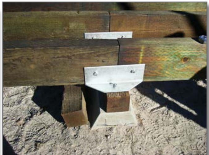
Step 10—Where steel pipes are not needed, a 1/4-inch thick neoprene pad is placed between the foundation block and beams to keep moisture away from the wood beams.
