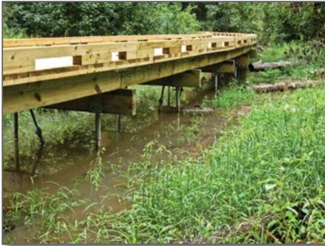
Figure 2—This elevated boardwalk on the Town Creek Off-Highway Vehicle (OHV) Trail system at the Chattahoochee-Oconee National Forest in Georgia is supported by helical piles.
