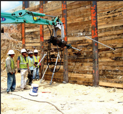
Soldier Pile & Lagging Shoring
